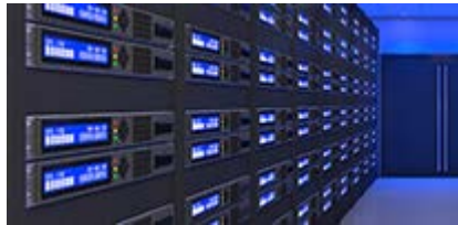
Uninterruptible power supplies
