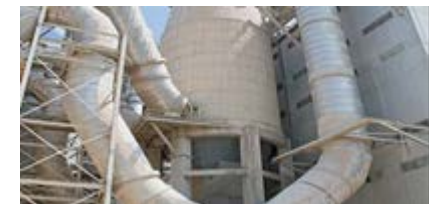
High voltage motors
